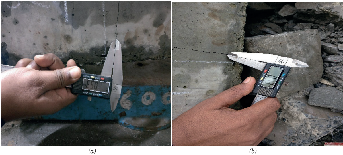
Figure 13 Crack behavior of RC beam with Fe-SMA reinforcement (a) at maximum deflection (b) recentering of RC beam with Fe-SMA reinforcement after unloading
