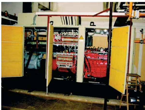
Fig. 1 Combined cogeneration unit
